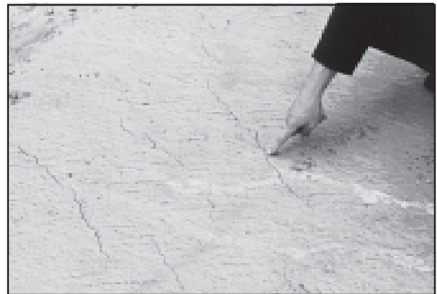
Plastic Shrinkage Cracks
